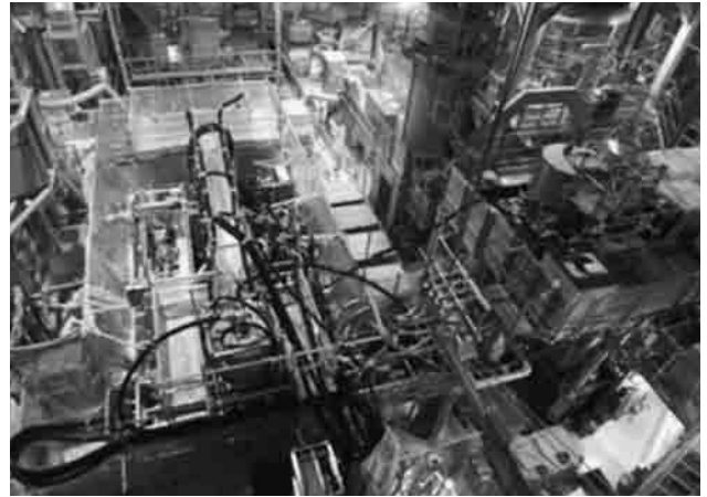
Fig. 10 View of auxiliary systems for FSD in Mihama Unit 1
